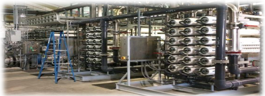
Example of an operational reverse osmosis facility
