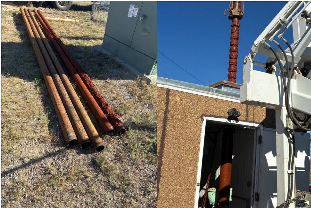
(Well 17 malfunctioned recently due to lightning strike. The level of oxidation on the lower pipes is more than usual, but not a concern.)
